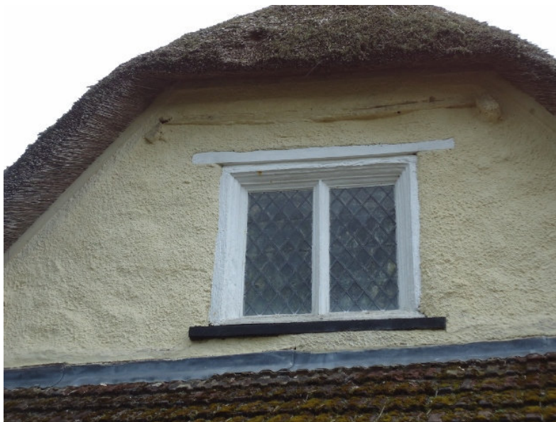
Photograph 4 - 16/17 Century ovolo moulded window
