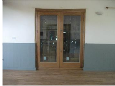
Old barn door exposed and seal with internal glazed doors to enable viewing
