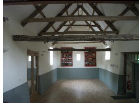
South-facing showing A-frame roof construction a feature of the original barn dating to late C17th
