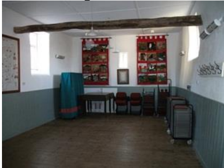
South-facing showing asbestos based ceiling hiding original features of the roof structure.
