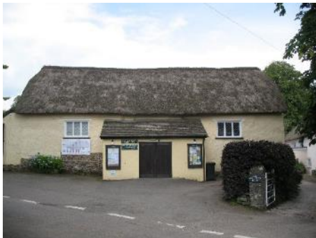
External view of the front of the Hall showing the need for the periodic renewal of the thatched roof
