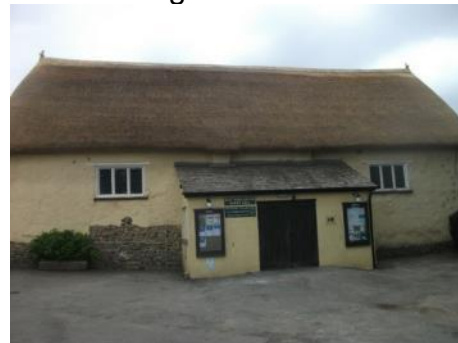
The thatched roof of the Hall following the work undertaken by the Master Thatcher.
