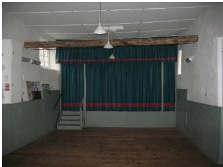
North-facing showing asbestos based ceiling hiding original features of the roof structure.
